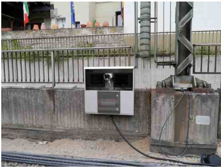
Installed MOVIE System
